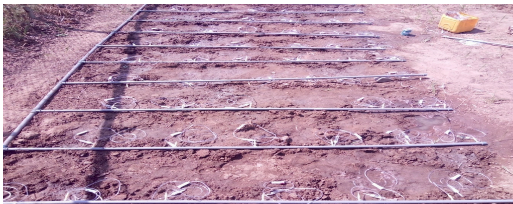
Plate 1: Experimental Set-up of PVC pipes and Medi-emitters
