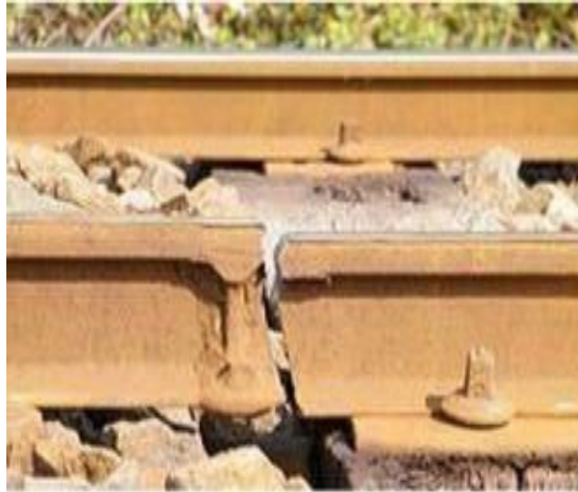
Fig. 1 Railway crack on track
