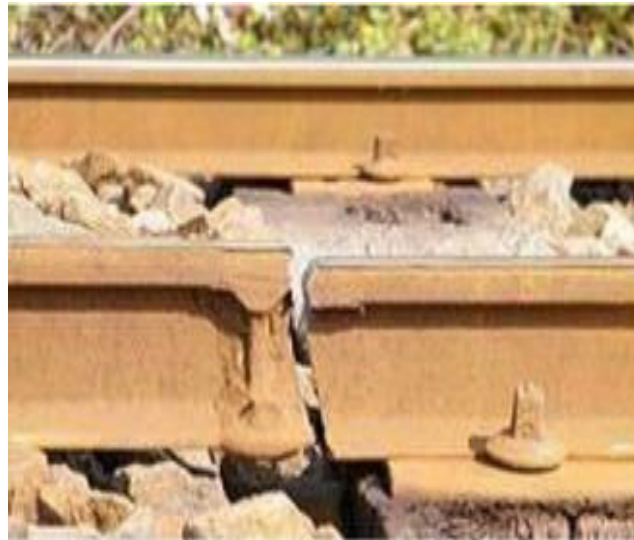
Fig. 1 Railway crack on track
