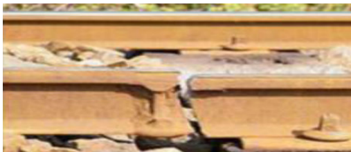
Fig. 1 Railway Track Crack
