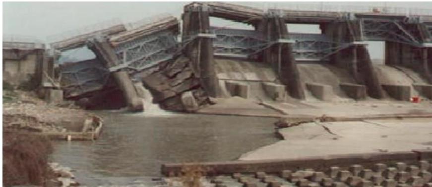
Fig. 4 Failure in the spillway of Shih-Kang Dam [8]
