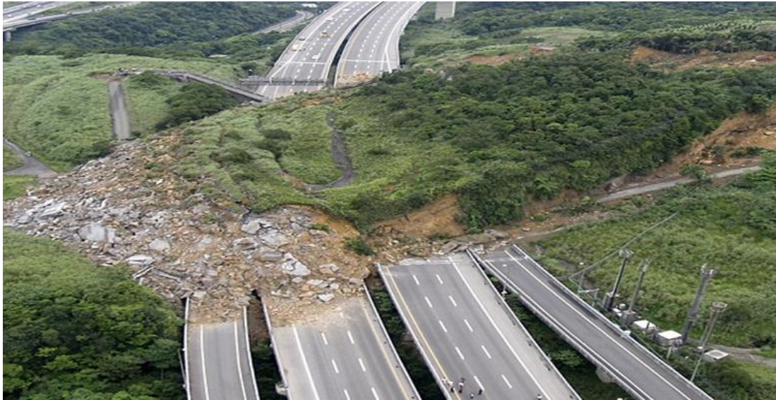
Fig. 1 Slope failure on motorway No. 3 of Taiwan (2010). For the removal of the soil, 50 excavators, 100 trucks and 1000 workers had to be used for 20 days [5]
