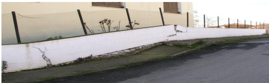
Fig. 7 Cracking on road surface and a house courtyard [16, 17]
