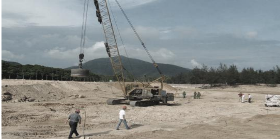
Fig. 8 Application of the dynamic compaction method, which consists of dropping large weights onto the ground [20]
