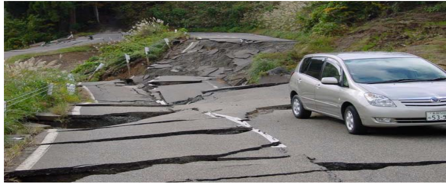
Fig. 3 Road destruction in the Nigata-Ken Chuetsu (Japan) earthquake [7]
