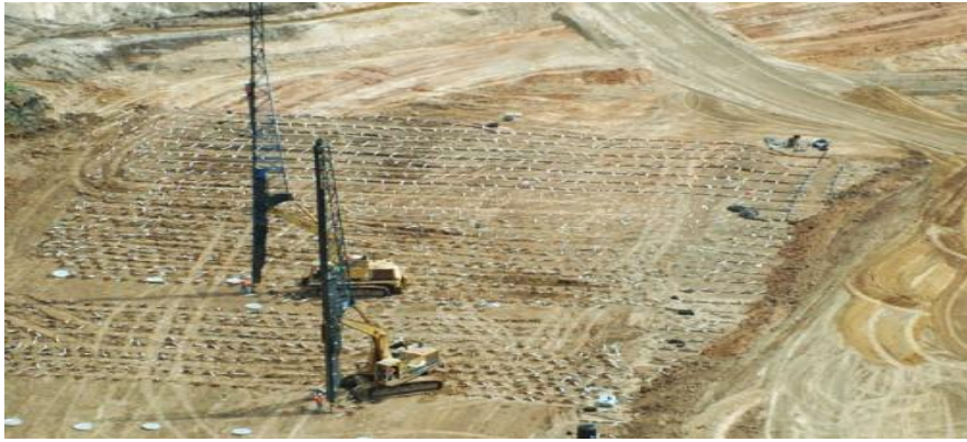
Fig. 9 Geocomplex vertical drains are placed in the ground by using a special crane with a vertical guide, in close intervals between distances of 2-4 m [20]
