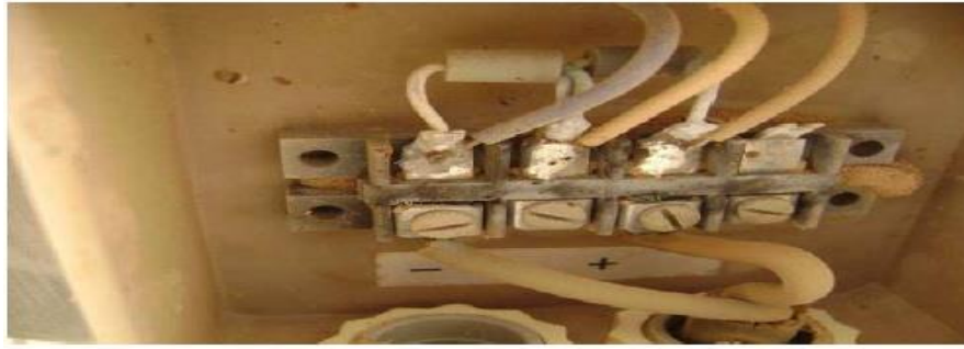
Fig. 5: Discoloration of the junction box
